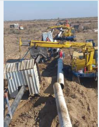
EBS PETROLEUM · 2019 S1 Block Oil Trunk Line & Flow Line EPCC delivery at Nahrawan, Baghdad · $3.81M
